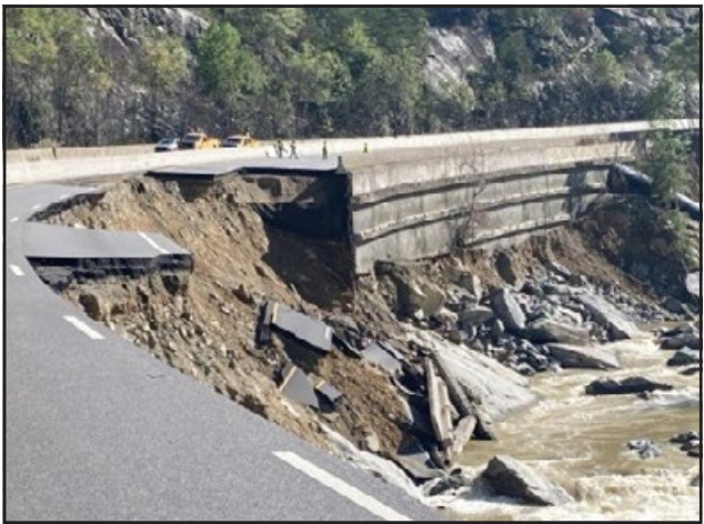
Photo provided by Sharon McMahon It's been two years since our columnist witnessed Hurricane Helene's devastating power. Here you see a part of Interstate 40 washed away in western North Carolina.
