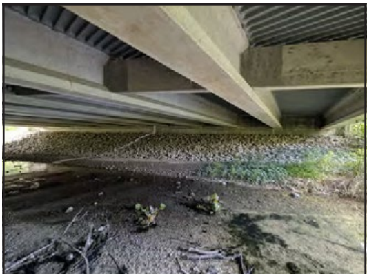
Photos provided by USI Consultants
