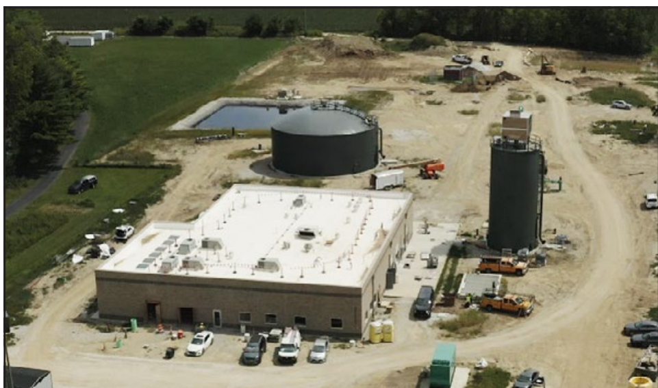
Photo courtesy Indiana American Water A birds-eye view of Indiana American Water's new water treatment plant in Sheridan, taken during construction in October 2024. The new water treatment plant is located in northeast Sheridan, near the high school.
