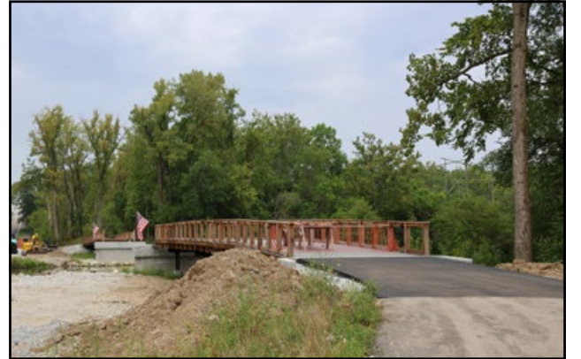
Photo provided by Hamilton County Parks & Recreation Preliminary work for the placement of Bell Ford Bridge is underway at Geist Park.
