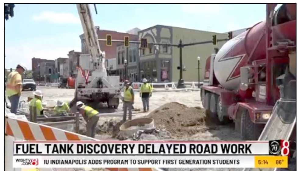
INDOT said work underway now should finish during the first week of August.
